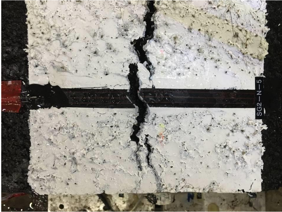
Fig 4 North section surface crack reached inner vertical edge
