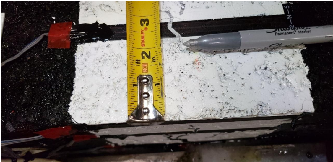
Fig 4 North section surface crack 2 inch from the inner vertical edge
