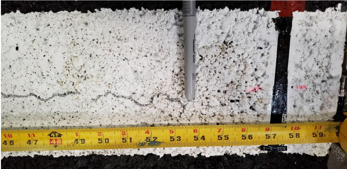
Fig 7 South section surface crack 6 inches from the outer vertical edge
