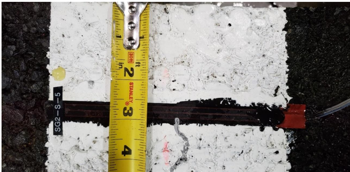
Fig 6 South section surface crack 3 inches from the inner vertical edge
