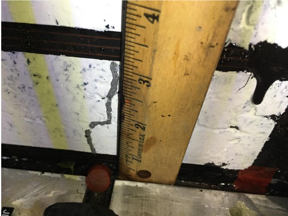
Fig 5 Bottom-up crack at SG6-S-0 3 inch long
