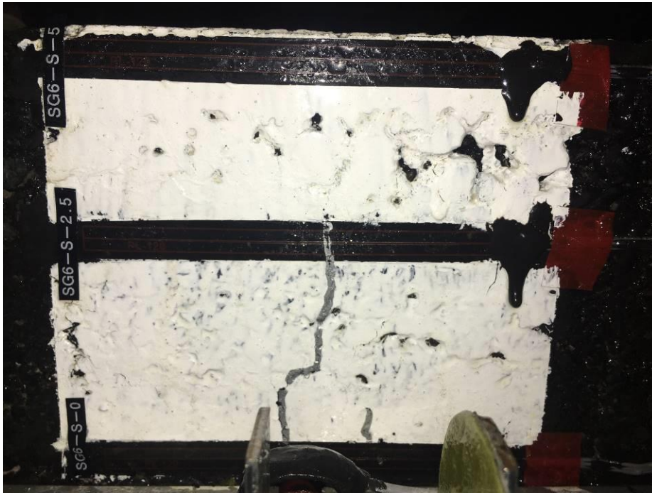
Fig 6 Bottom-up crack at SG6-S-0, SG6-S-2.5 approximately 3.5 inch long
