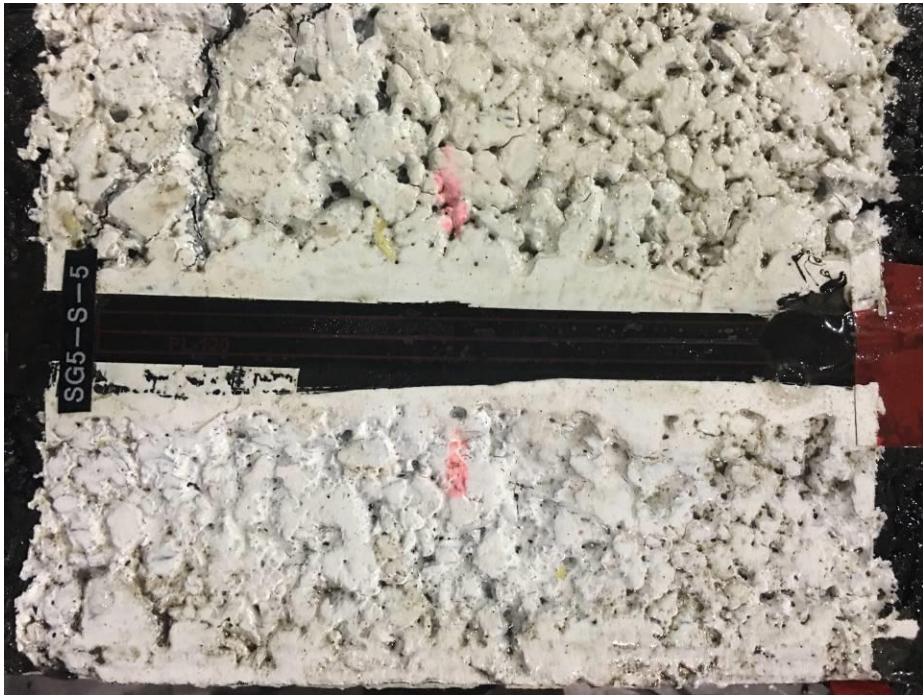
Fig 8 South section surface crack 3 inches from the outer vertical edge
