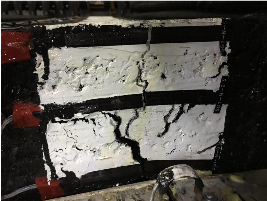
Fig 1 Bottom-up crack at north section inner vertical edge reached top surface
