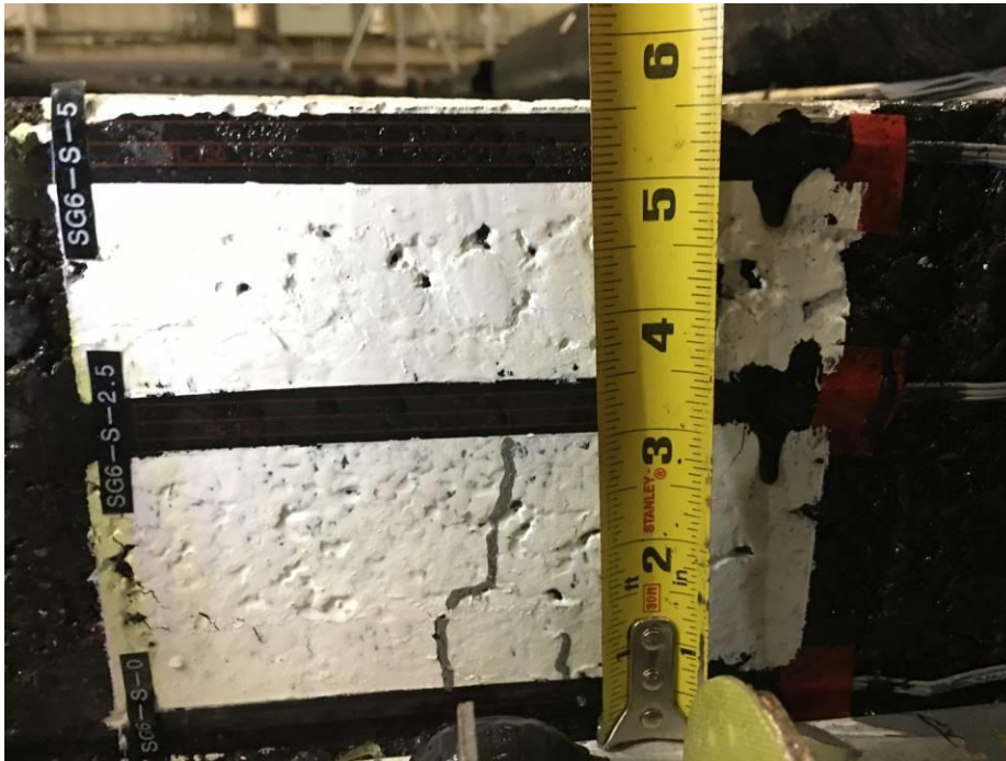
Fig 6 Bottom-up crack at SG6-S-0 3 inch long
